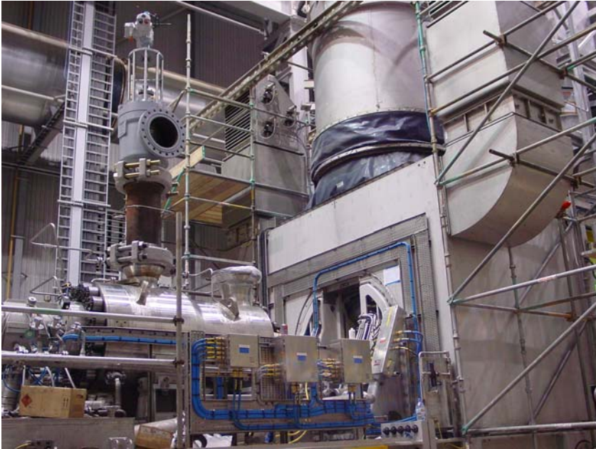
Figure 7.26 27 MW gas turbine for injection pump drive. The complete set on the test bed in Leeds/UK
